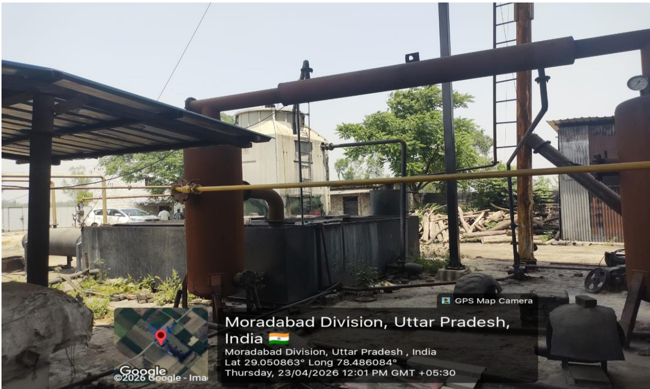
After generation of pyro gas, the same is to be used for the purpose of heating reactor along with alkaline scrubber with mist eliminator attached.
