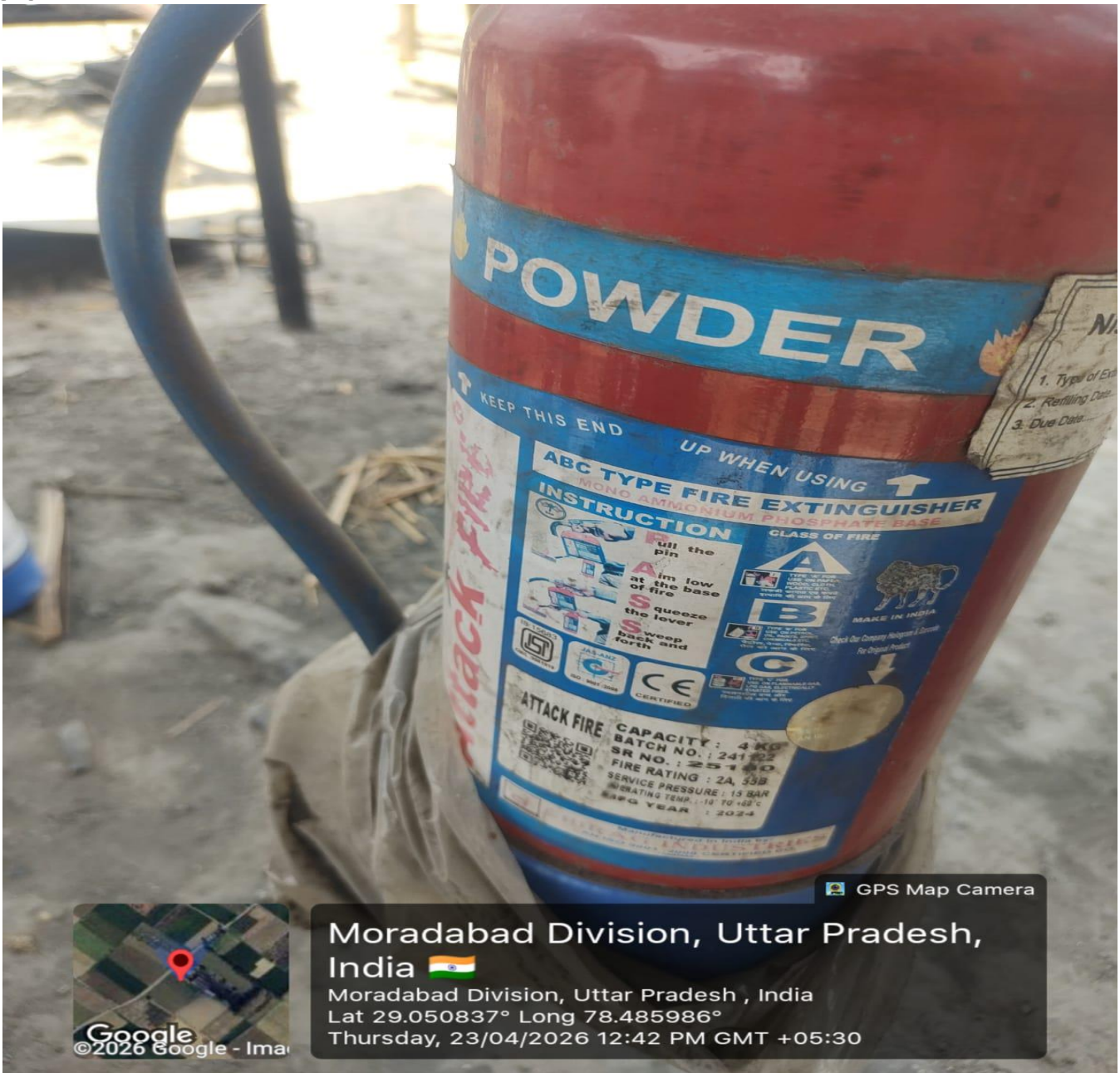
ABC type Fire Hydrant
