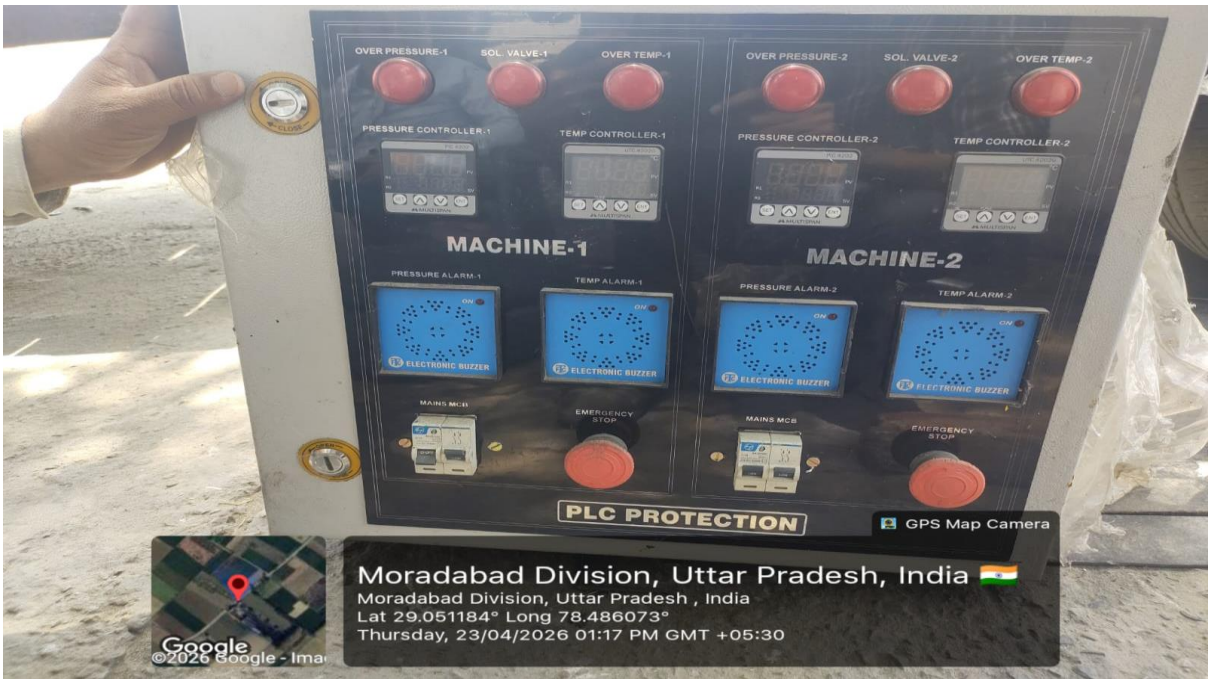
Programme Logic Controller (PLC) based system for control – not installed
