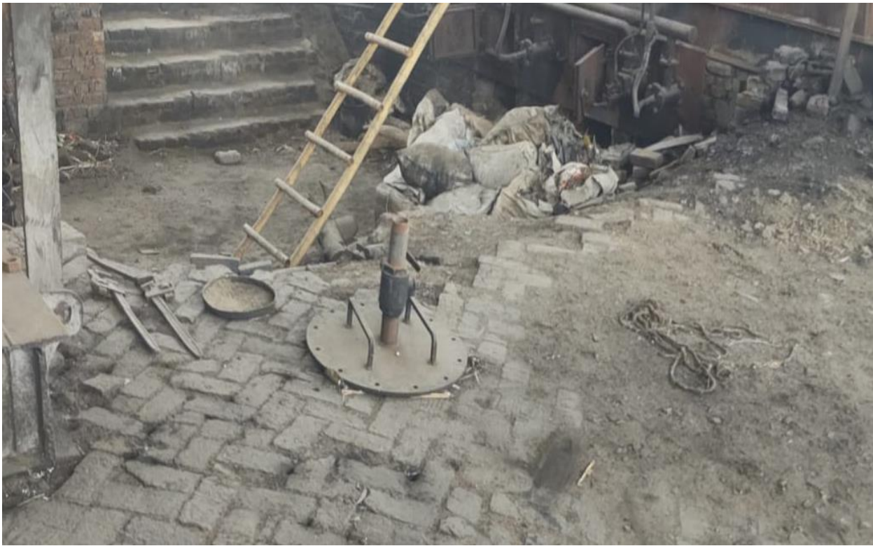
Temporary arrangement of Nitrogen purging system.
